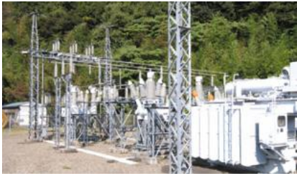
Substations and power stations
